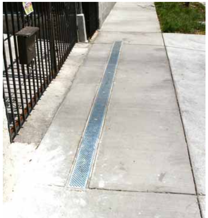
Metal grating captures runoff from the driveway.
