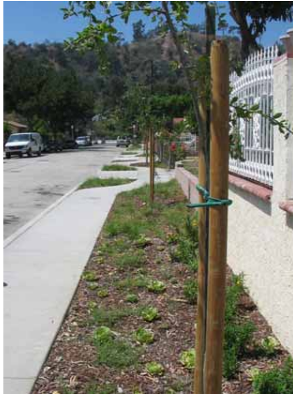
Perforated pipes below the soil and plants collect rainwater.
