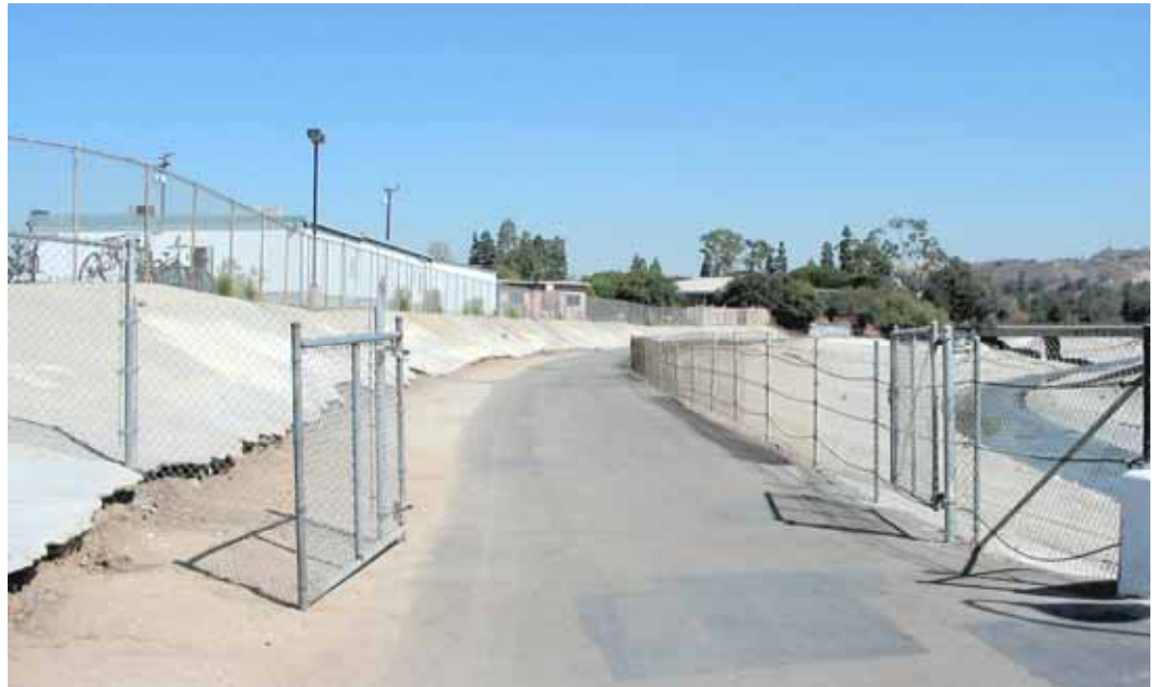
A current view shows chain link fencing and barren, eroding sprayed concrete banks.
